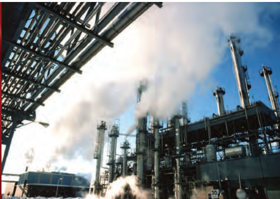
Instrumentation and Automated Pneumatic Controls
